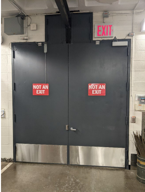
Figure 6: The Loading Dock Entrance (Not an Exit)
