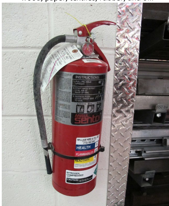
Figure 14: ABC Fire Extinguisher with the typical small spray nozzle
